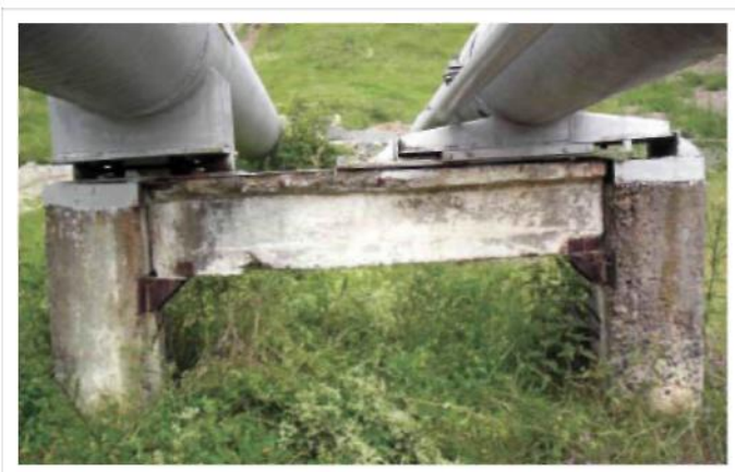
Fig. 5. Overall view of the mounting group of the oil pipeline with the D = 720 mm, whose frame is leaned onto the riser and girder.
