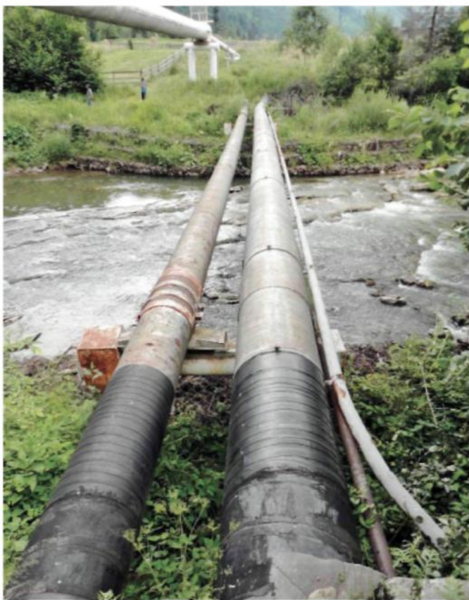
Fig. 1. Overall view of aboveground passages of “Druzhba” oil pipelines through the Oriava river
