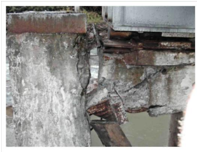
Fig. 2. Destruction of the mounting group of the second oil pipeline support D = 720 mm
